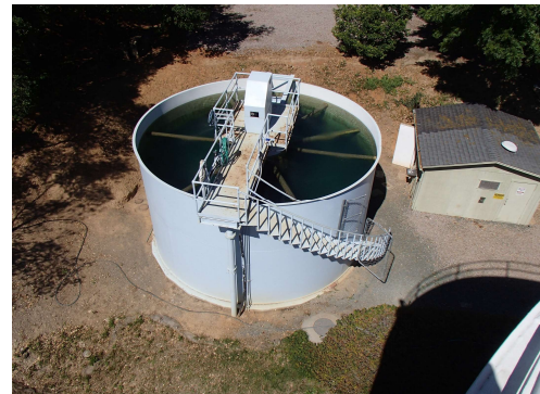
Coagulant for sedimentation in tank
